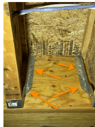
Missing fasteners (nails)
