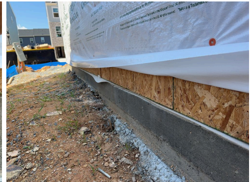
Foam sill sealer pushed out
