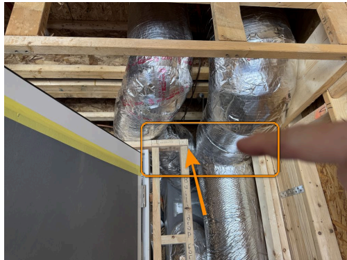
Utility room wall framing cut
