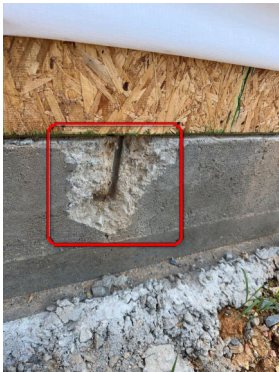
Broken concrete with anchor bolt missing
