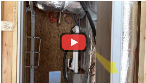
Garage Utility room wall framing cut
