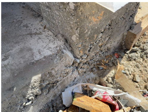
Honeycombing to the right of garage of foundation wall
