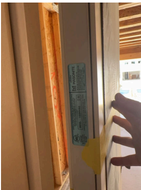
Fire rated utility door
