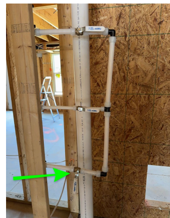
Main Water Shutoff
