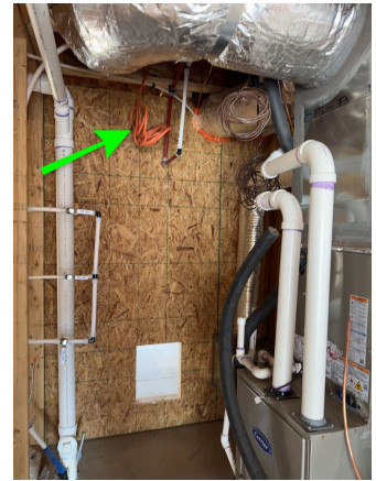
Electrical for planned water heater
