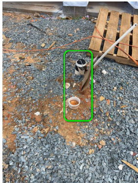
driveway drain cleanouts
