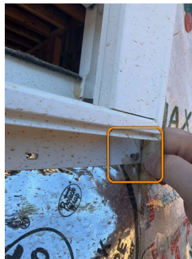
Proper placement, but underdriven fastener.
