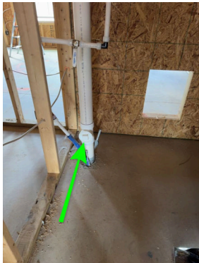
Utility room cleanout
