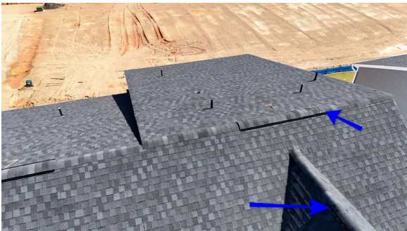
Fasteners (nails) exposed
