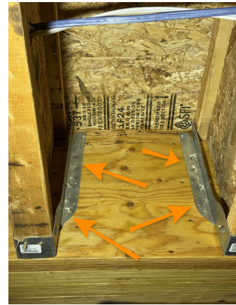
Missing fasteners (nails)
