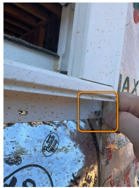
Proper placement, but underdriven fastener.
