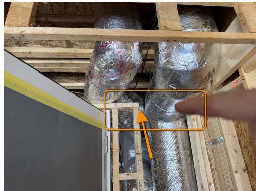
Utility room wall framing cut
